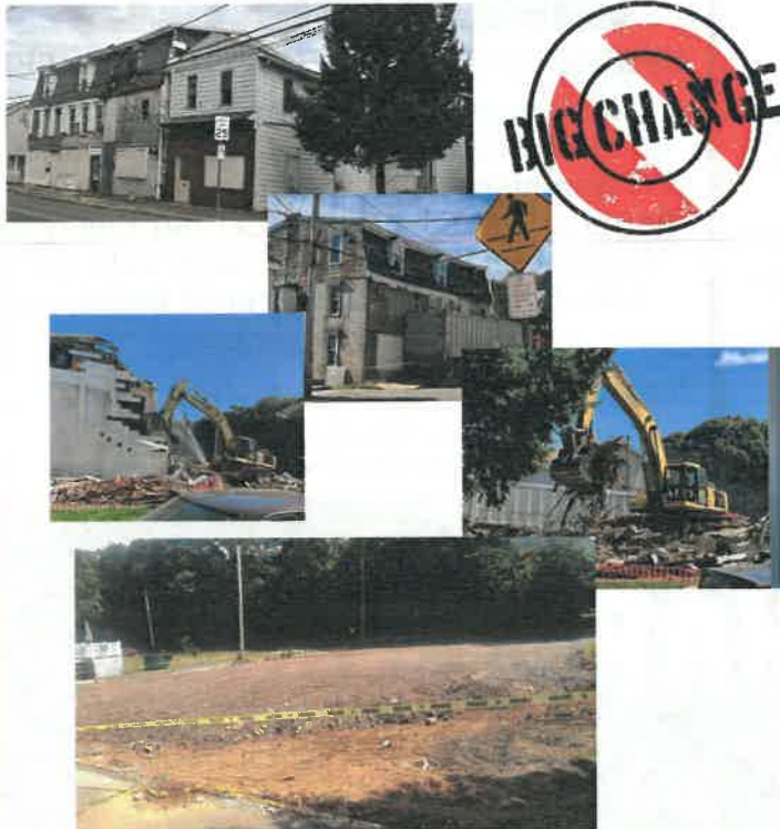
18-28 North Market Street have been demolished and the property will be made into a Municipal parking lot
